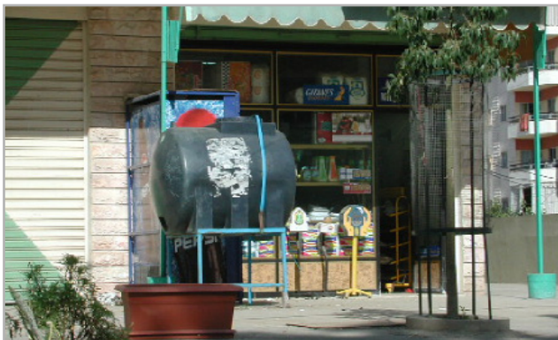
Water tanks within shops
